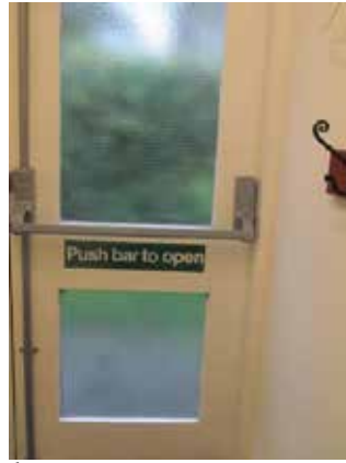
push bar to open emergency exit door.jpg
