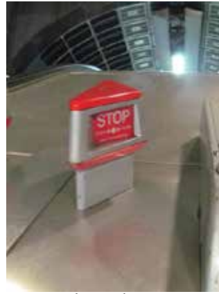
underground escalator emergency stop button.jpg
